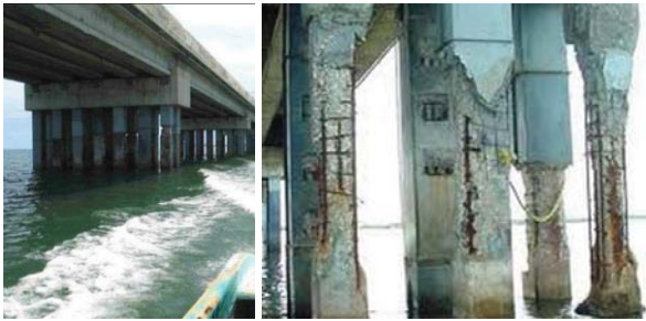
Figure 2. Typical pathologies of the existing bridge
